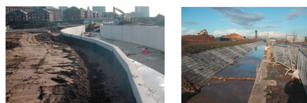
Several views of the new canal under construction. Above and right is the route through the old central docks, with Salthouse Dock top right.
